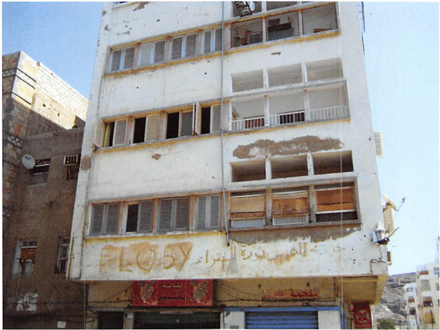
FLOSY slogan ('Liberation Front...Revolution for the Poor') preserved on a building in Aydarus Street, Crater, Aden.
