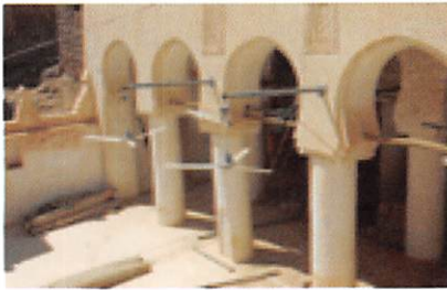
View of east facing arcade from courtyard with scaffolding to reinforce the vaults.
